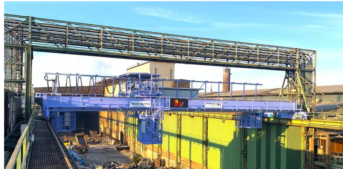
Replacement of high alloy scrap handling crane at Witten. The capacity has been increased to 16 t and the crane break system has been equipped with a modern energy recovery system.
