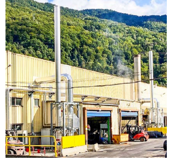
District heating at Ugine
