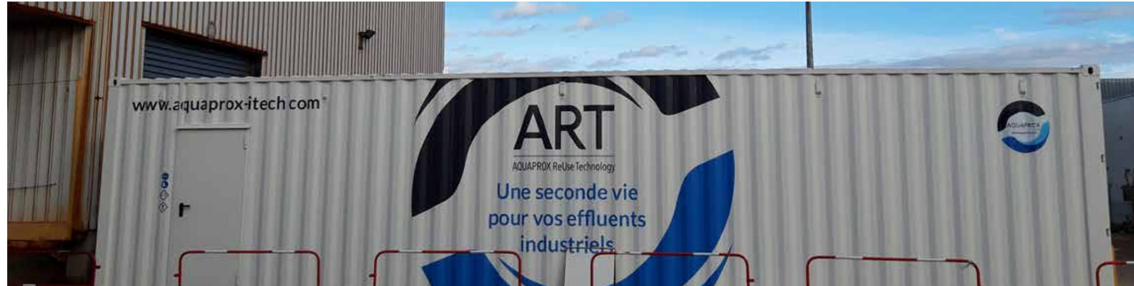
Process water recycling in Bourg-en-Bresse
