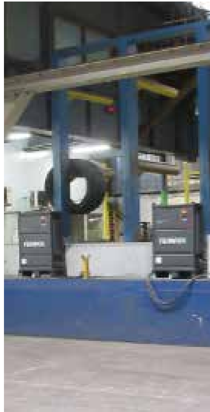
Electric charging stations for vehicles
