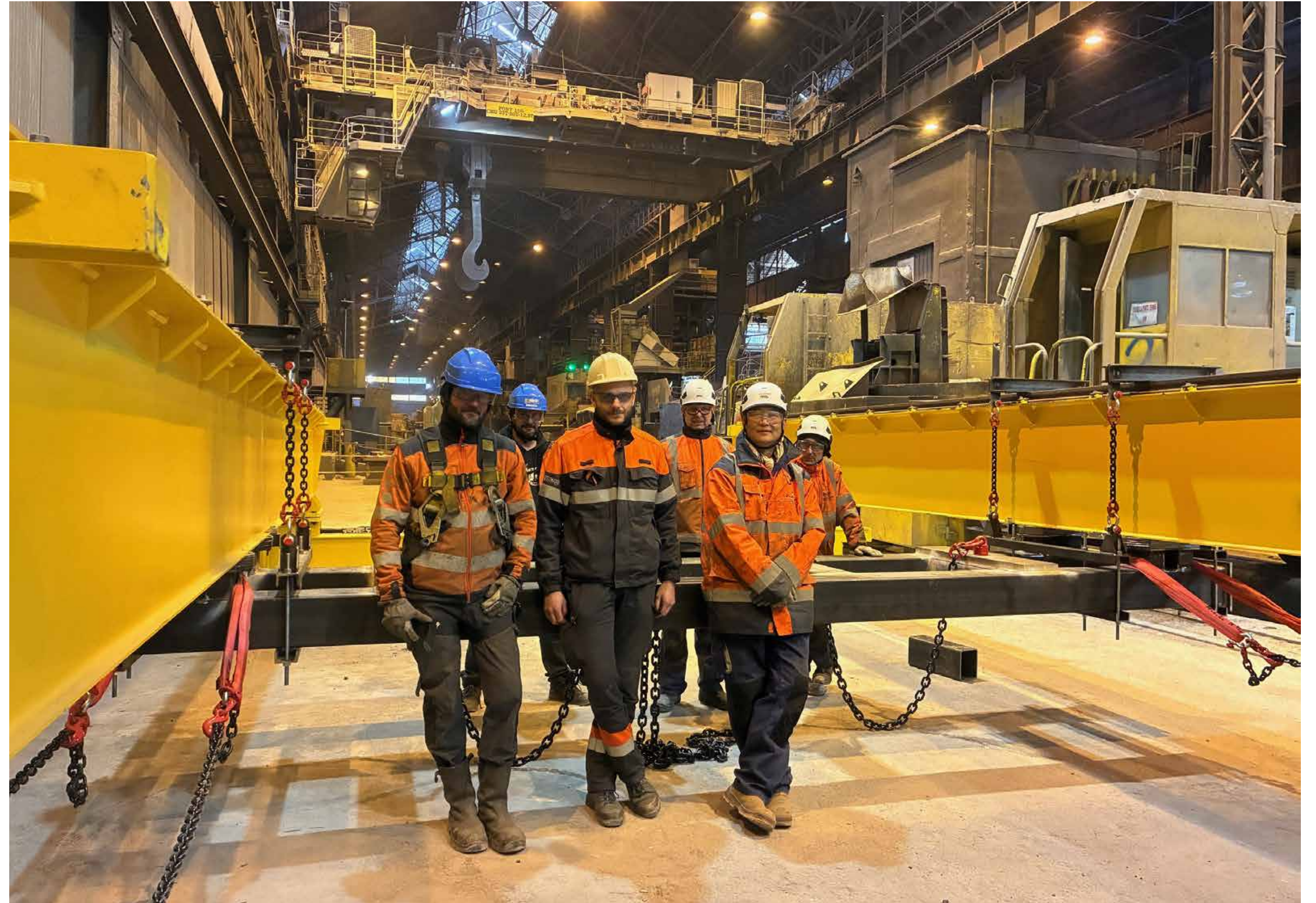
Replacement of a bridge at the steel mill in collaboration with SECAL
